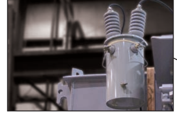
CT's (Bushing mounted internally)
